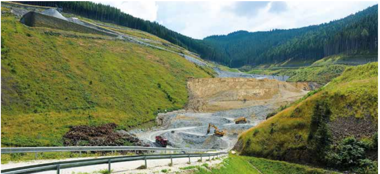
Longsgraben disposal site during the Semmering Base Tunnel excavation (photo courtesy of Austrian Federal Railways © ÖBB/Ebner)
