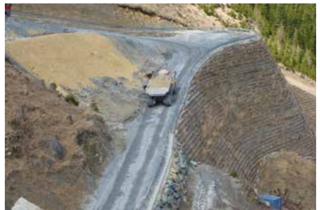
Figure 7: Adding quantities of soil to widen the access road resulted in a sudden rise in strain behind the structure
