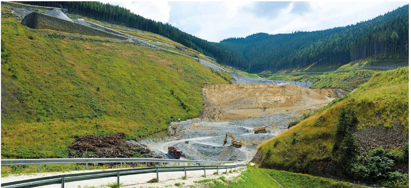
Longsgraben disposal site during the Semmering Base Tunnel excavation (photo courtesy Austrian Federal Railways © ÖBB/Ebner)
