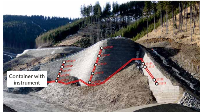
Figure 4: The geogrid and sensing cables were deployed within the earth retaining structure
