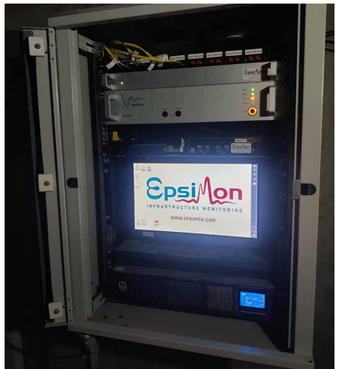
Figure 3: In the basement, the rack-mounted instrumentation comprises the fibrisTerre distributed fiber optic sensing interrogator, switch, computer, and accessories.
